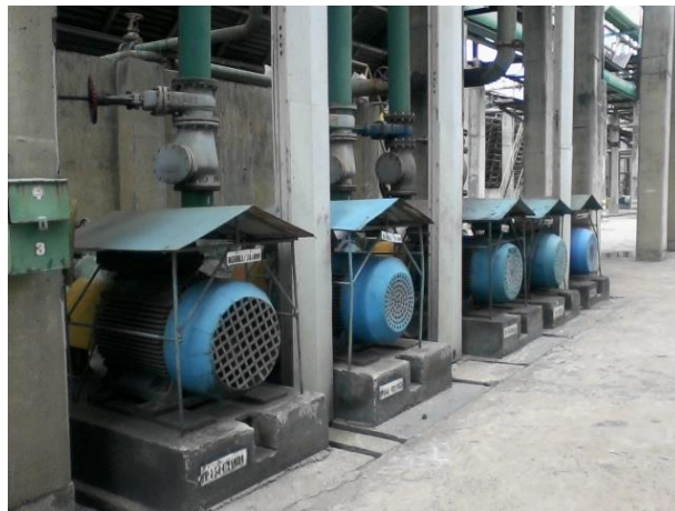
Gambar 2.46 Cooling Tower Pump
